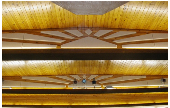
Ceiling beams with acoustics, facing speaker
